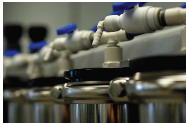
Membrane test ports for isolation profiling
